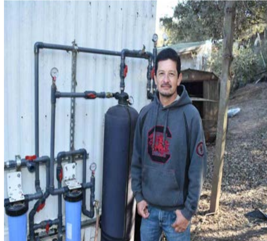
Community Partner Roberto Ramirez pictured next to the Phase 2B treatment system installed at DWMC-14 located near Royal Oaks in north Monterey County. This treatment system is the 3.6 cubic foot size. 12
