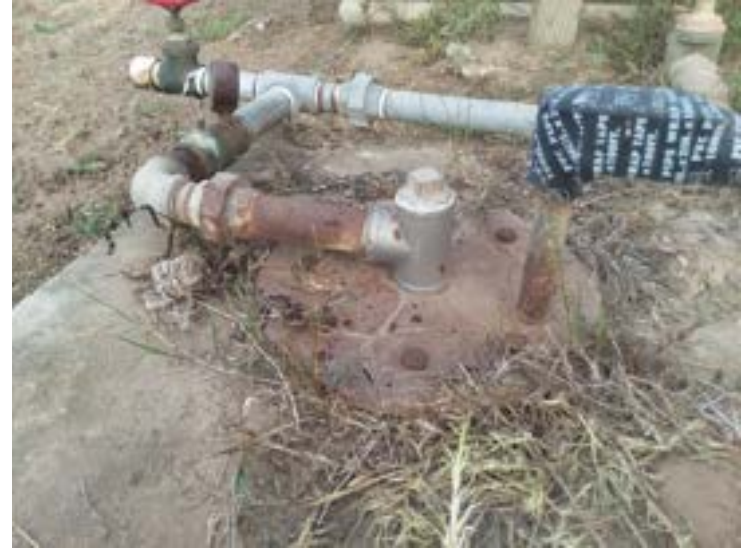
Cracked well seal at potential pilot project location. Photo by Weber Hayes and Associates.
