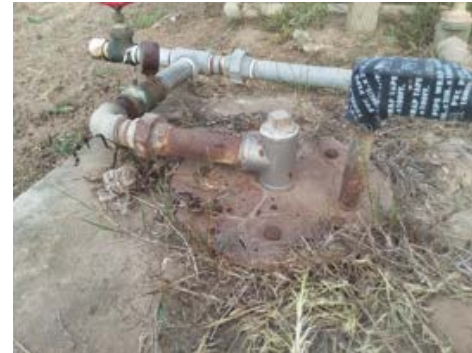
Cracked well seal at potential pilot project location. Photo by Weber Hayes and Associates.
