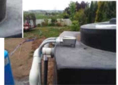
DWMC02 - Replaced Junction Box at Tank for Float Switch and Ozonator
