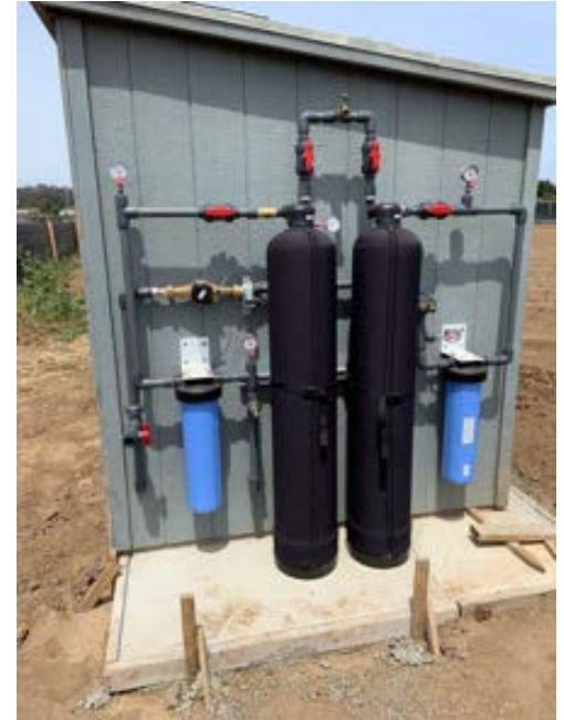
Phase 2B treatment system installed at DWMC-21 located near Moss Landing in north Monterey County.
